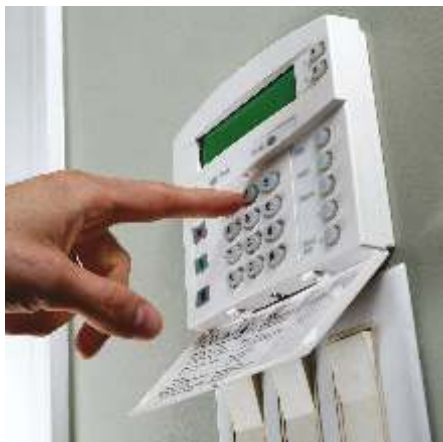
SECURITY ALARM SYSTEM
