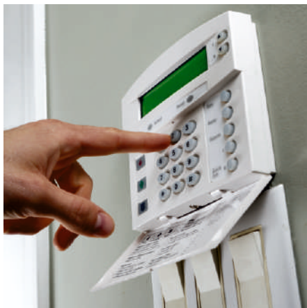
SECURITY ALARM SYSTEM
